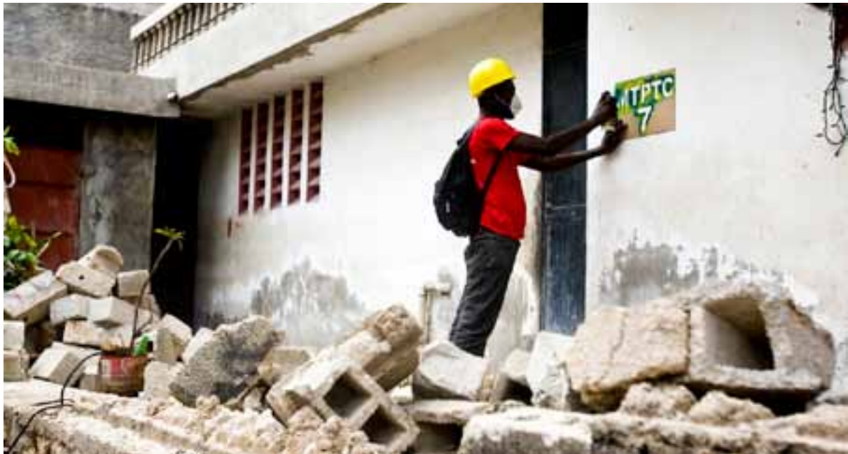
A worker in Haiti marking the results of a structural assessment on an earthquake-affected building in a Ministry of Public Works project financed by the Global Facility for Disaster Reduction and Recovery and the World Bank.
