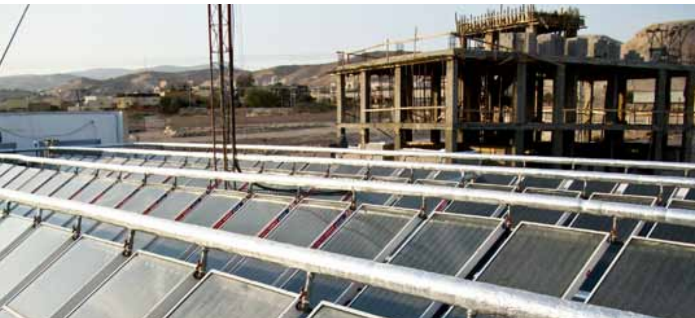
Solar power cells on the roof of the Jericho Police Training Facility, occupied Palestinian territory. UNOPS is implementing the project to build the facility for the Palestinian Civil Police, the EU Police Coordination Office for Palestinian Police Support, the European Commission and the governments of Canada, Denmark, Finland, the Netherlands, Sweden and the United Kingdom. Photo: UNOPS
