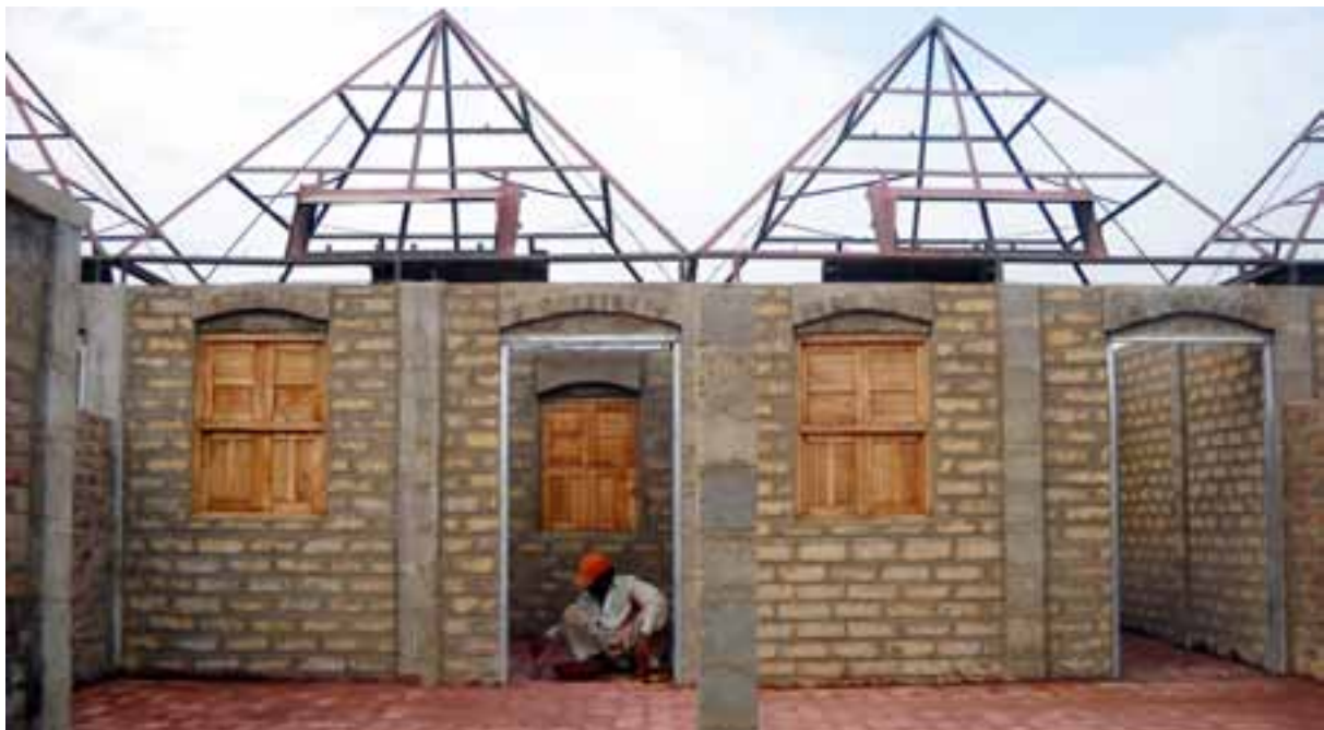
Energy efficient, environmentally sustainable houses being constructed in Pakistan's rural district of Thatta. The primary project was executed by UNOPS on behalf of the UNDP-GEF Small Grants Programme. Photo: Masood Lohar
