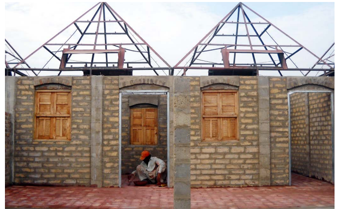
Energy efficient, environmentally sustainable houses being constructed in Pakistan's rural district of Thatta supported by the UNDP-GEF Small Grants Programme. Photo: Masood Lohar
